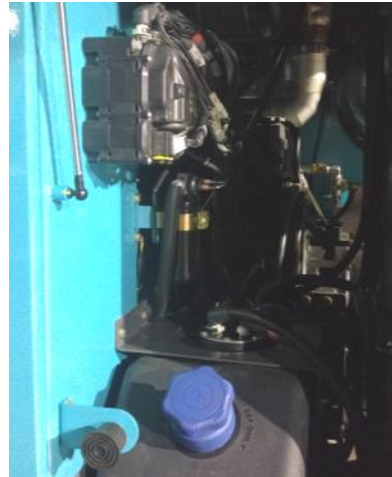
<Urea tank and pump>
