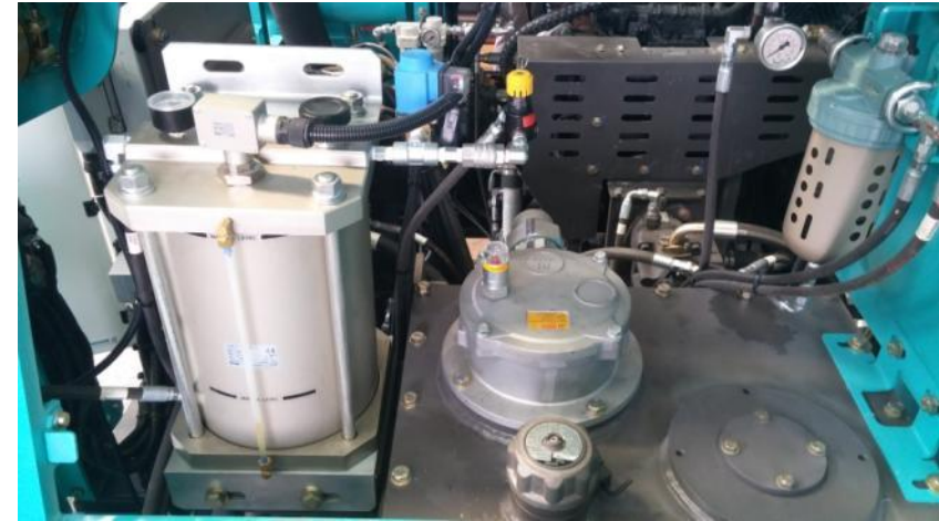
< Auto lubrication oil system>
